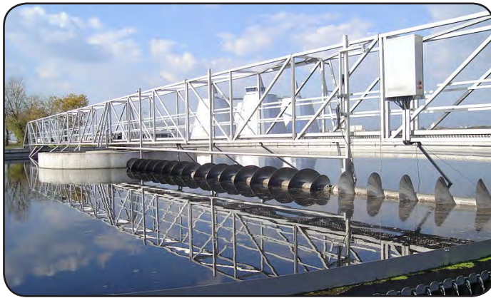
Wastewater treatment plants are vital for public health.
