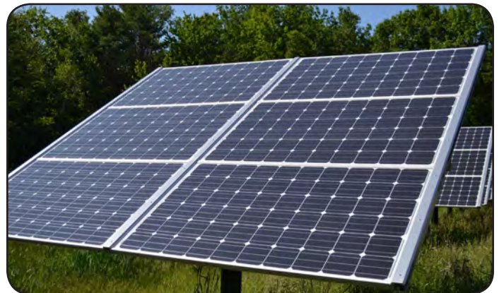
Solar panels array to produce energy for a municipal building. New Hampshire.
