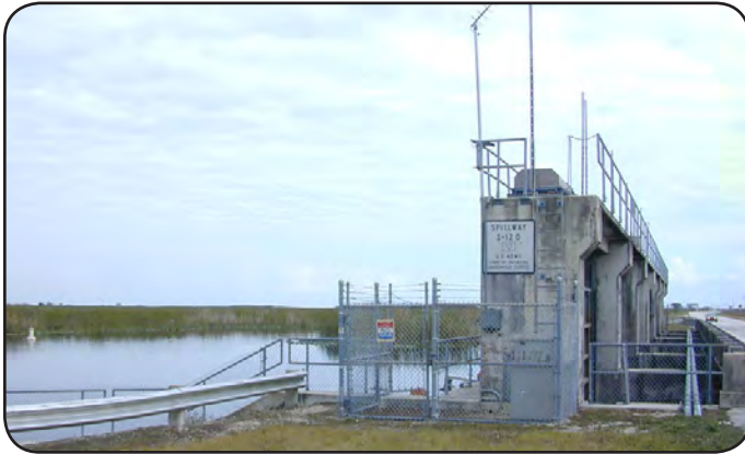
Water control structure on the Everglades.
