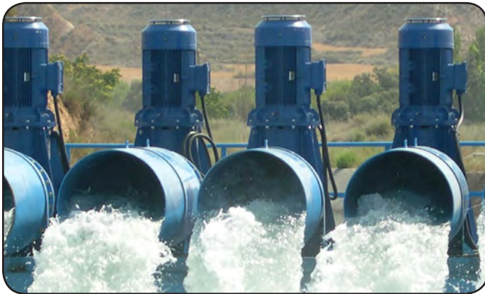
Outflow from a pump station
