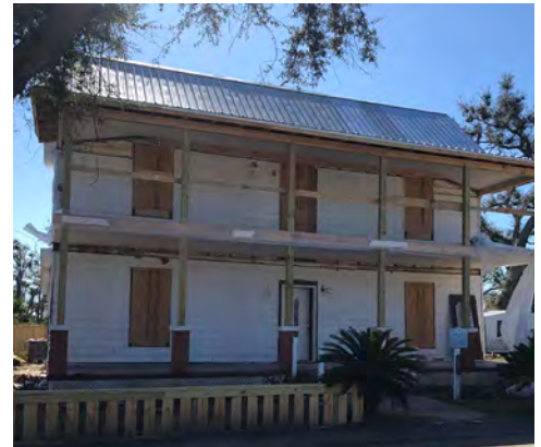
Stephenson Turner House, post-Hurricane
